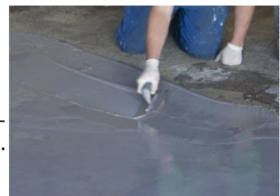
Spread the mixed material with a plasterers trowel or a long handled spreader.
