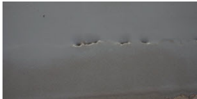
Fill holes and cracks to prevent the product from draining into voids and air bubbles rising to the surface.
